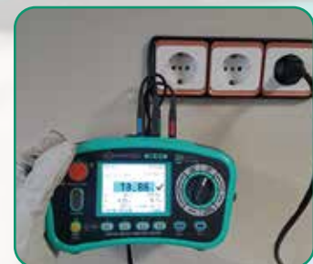
Loop test from a wall socket
