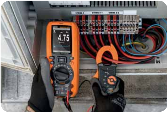
PV string Impp measurement.
