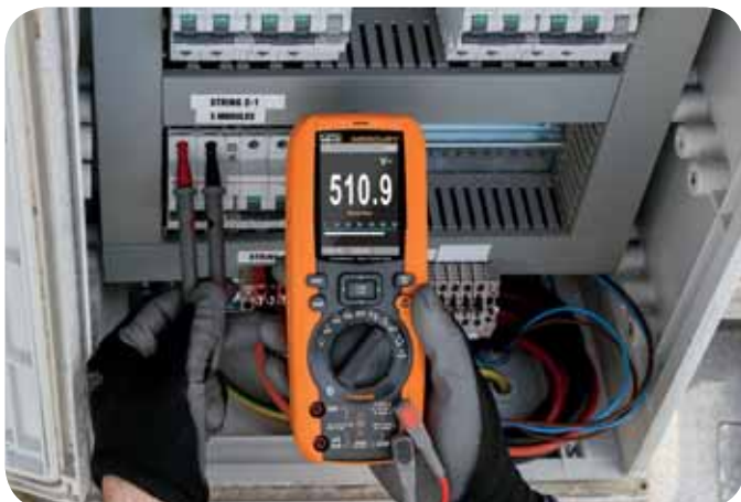
PV string Voc measurement
