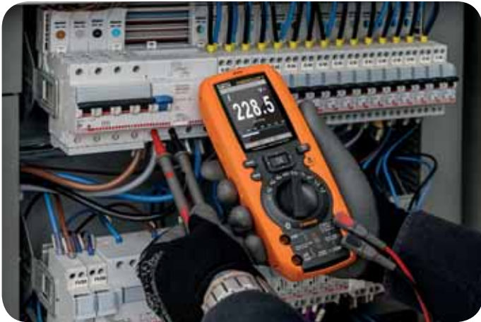
AC voltage measurement.
