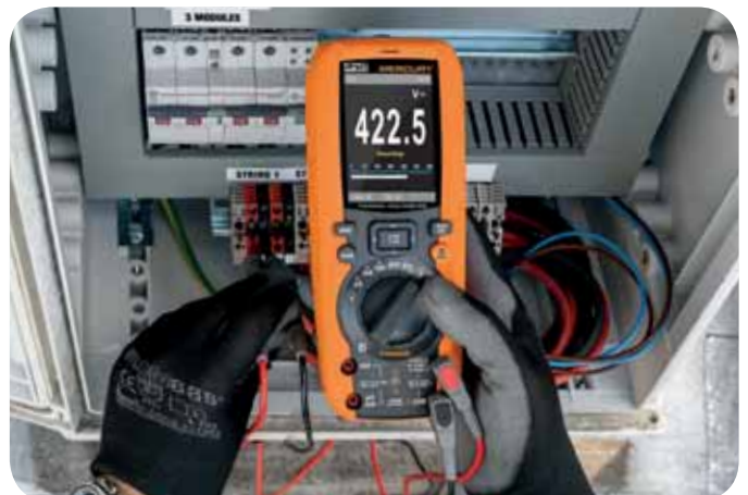
PV string Vmpp measurement
