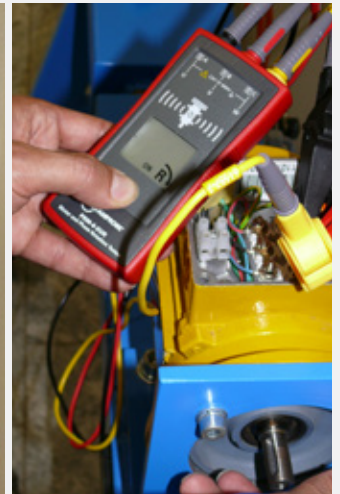
Check motor rotation prior to connection
